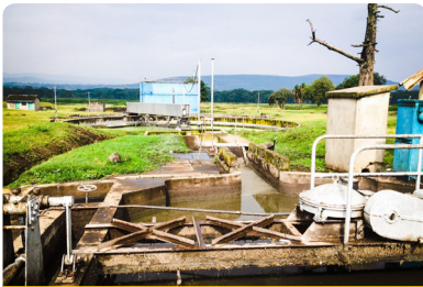
Wastewater treatment plant in Nakuru, Kenya.
